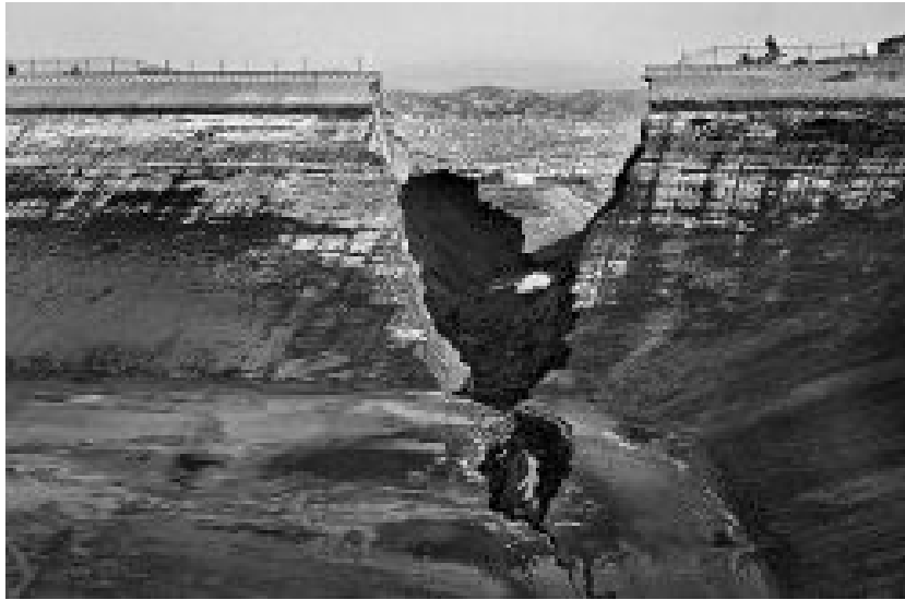
Fig 20: View from inside the reservoir of breach in Baldwin Hills Dam (Photo source: L.A. Times, December 15, 1963). (damfailures.org)
