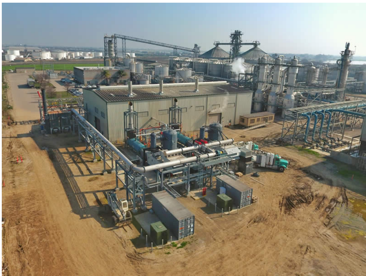
Figure 11. Pacific Ethanol facility located in Stockton. Processes ethyl alcohol that contains ammonia and flammable mixtures. Last RMP submission was made in 2013 while the last safety inspection date was in 2012. San Joaquin Elementary School is located 1.6 miles away. RMP source: https://rtk.rjfuture.org/rmp/facility/100000203665 Image source: https://www.pacificethanol.com/images/locations/stockton/stockton-facility-02.jpg
