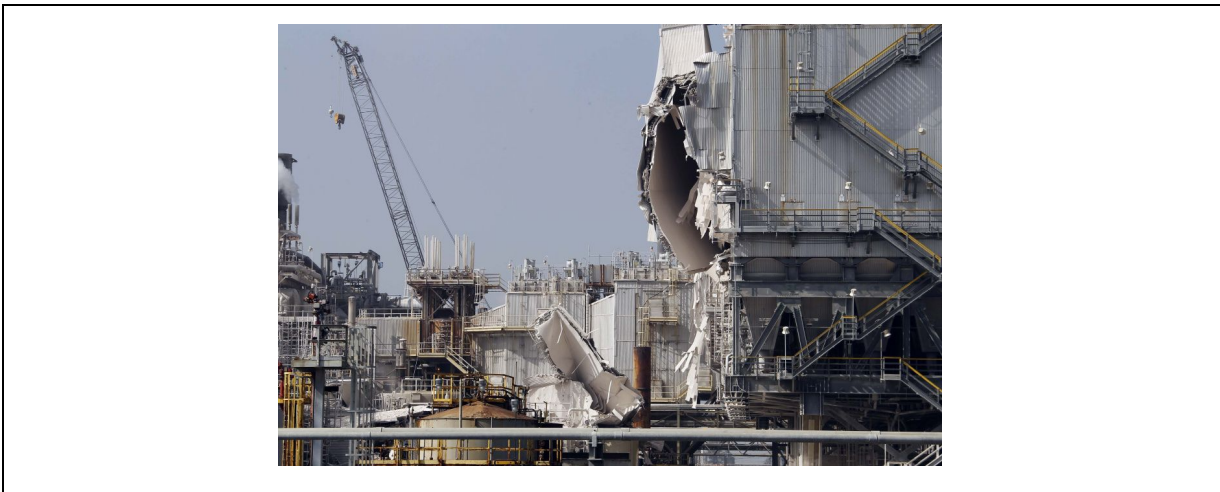
Fig 10: Due to the outdated equipment, the Torrance Refinery exploded. Taken from LA Times "Exxon Mobil's outdated equipment and procedures led to Torrance Explosion, Agency Says."
