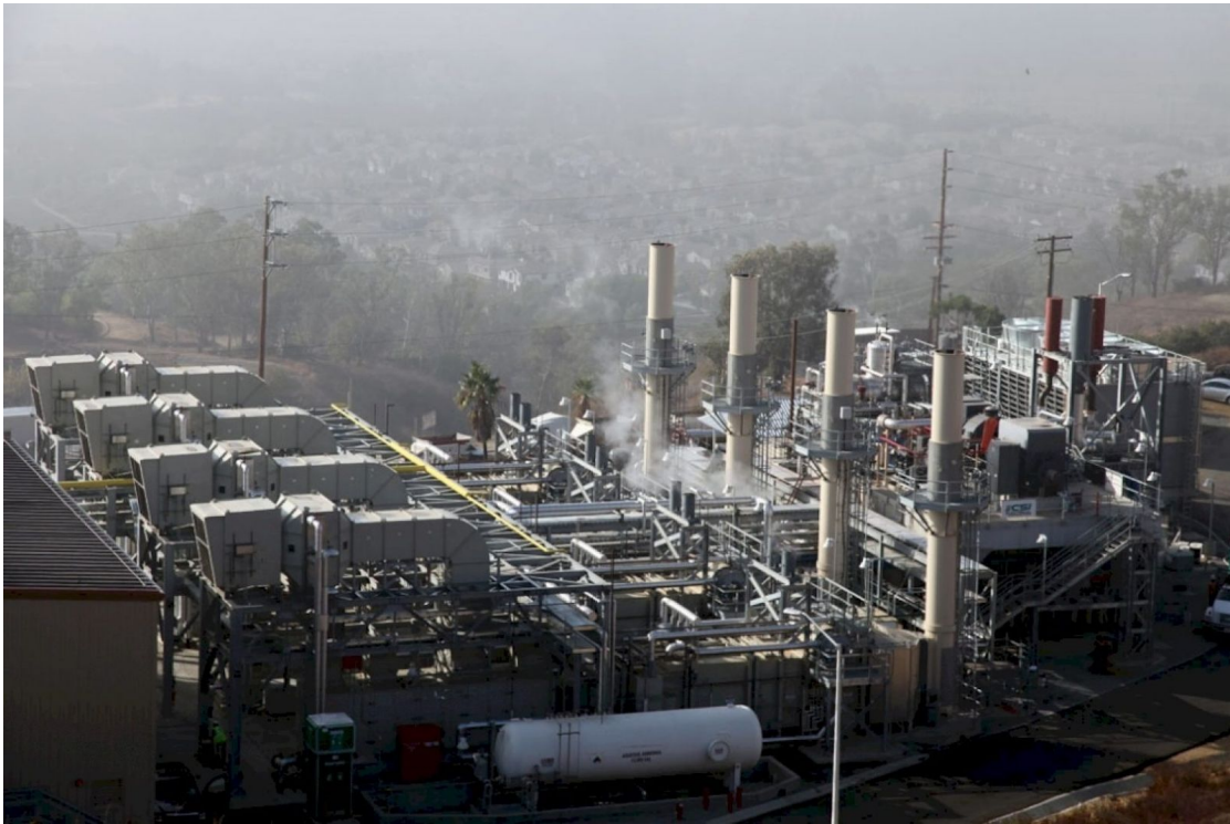
Figure 15. The Brea Power Plant, owned by Broadrock Renewables. The 2012 report claims the plant is producing greener energy using what they call “hot-dip galvanizing”, also used by a facility in the East Coast (American Galvanizers Association). It emits an unknown visible white gas as it generates power. (Photo from American Galvanizers Association 2012, retrieved July 15, 2020) Source: https://galvanizeit.org/project-gallery/brea-power-plant
